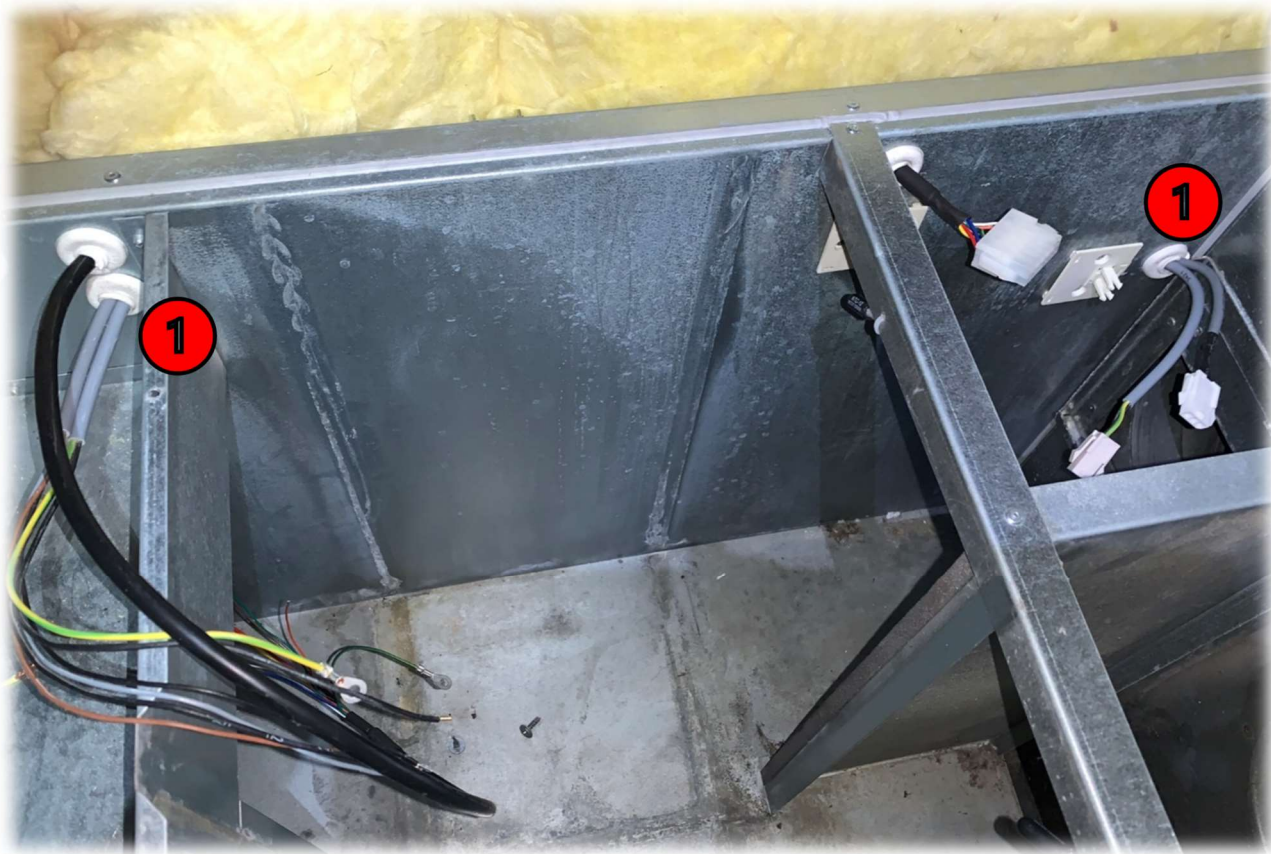
New extract air fan cables installed (1).
